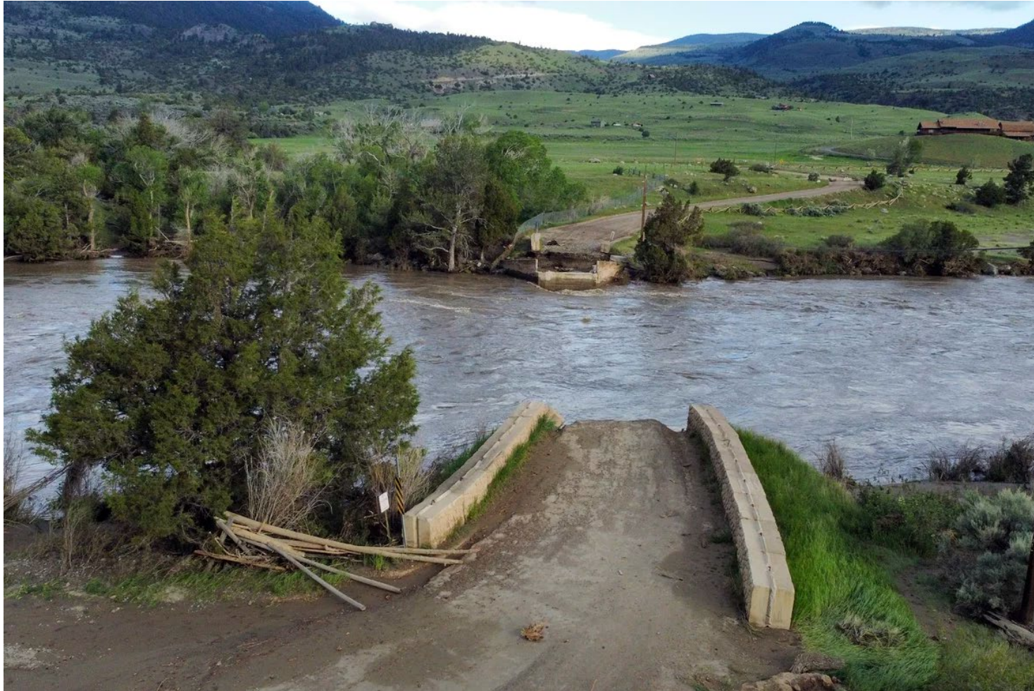
A washed out bridge shown along the Yellowstone River Wednesday, June 15, 2022, near Gardiner, Mont. Photo: Rick Bowmer/AP NPR
