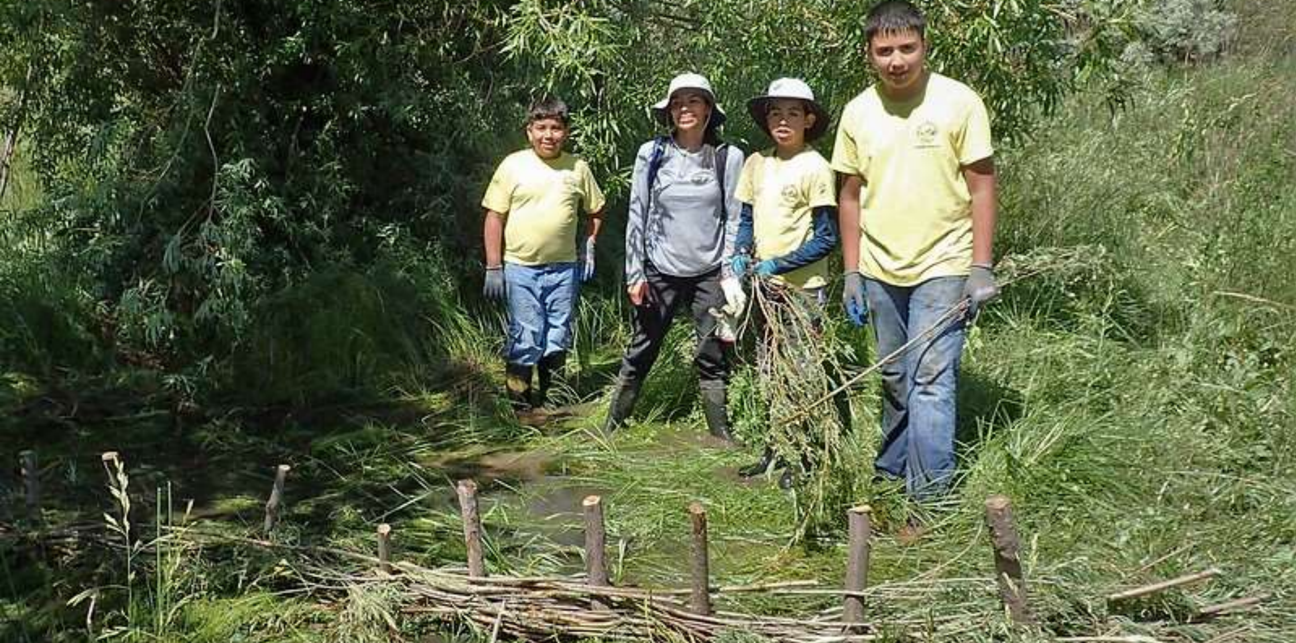
A beaver dam analog creates a wetland area (Boulder YSI, Wildlands Restoration Volunteers and CU-Outreach project)
