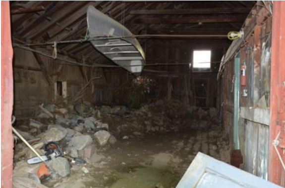
Figure 6. The inside of the barn after the flood. Part of the back wall caved in allowing the water to rush through with big boulders. My brother has cleared out part of it using his bobcat.
